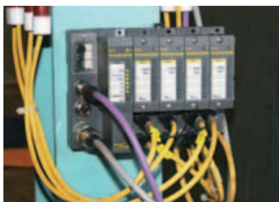
RFID modules are integrated into the automation network at Tower Automotive via the BL67 I/O system with PROFIBUS gateway
